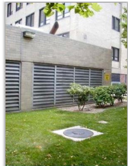
Figure 4-1. Air Intake Vent
